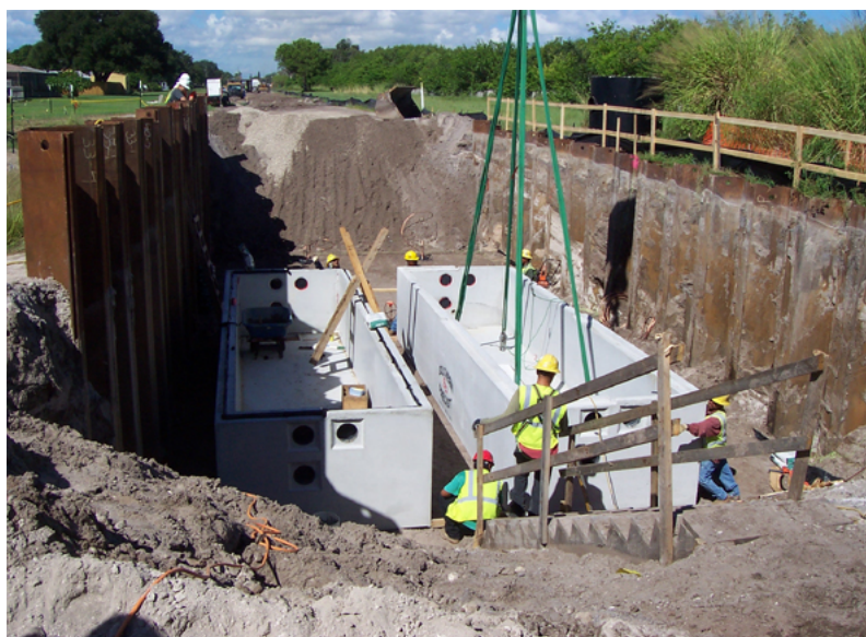
Figure BB-3-4. Typical XLPE Vault Installation
